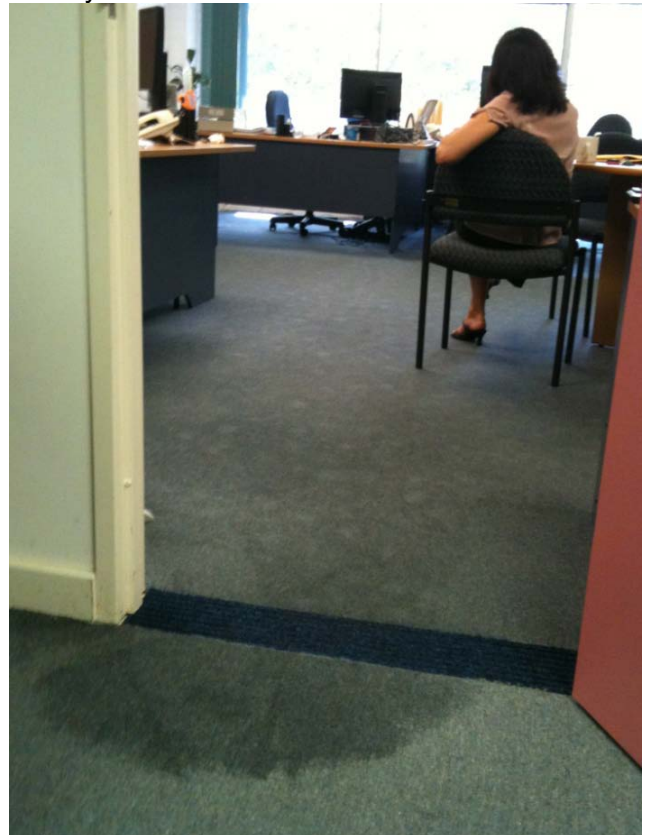
Water damage in the Shelter WA offices at Claisebrook Lotteries House
